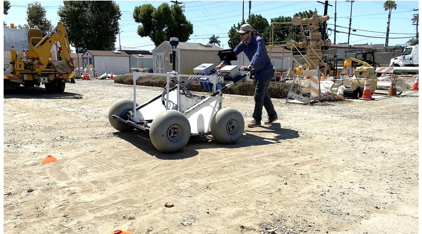
Enhanced Locating Technologies for Underground Pipelines with Better Accuracy (OTD 8.20.1)(CEC GFO-19-502, group 3)
