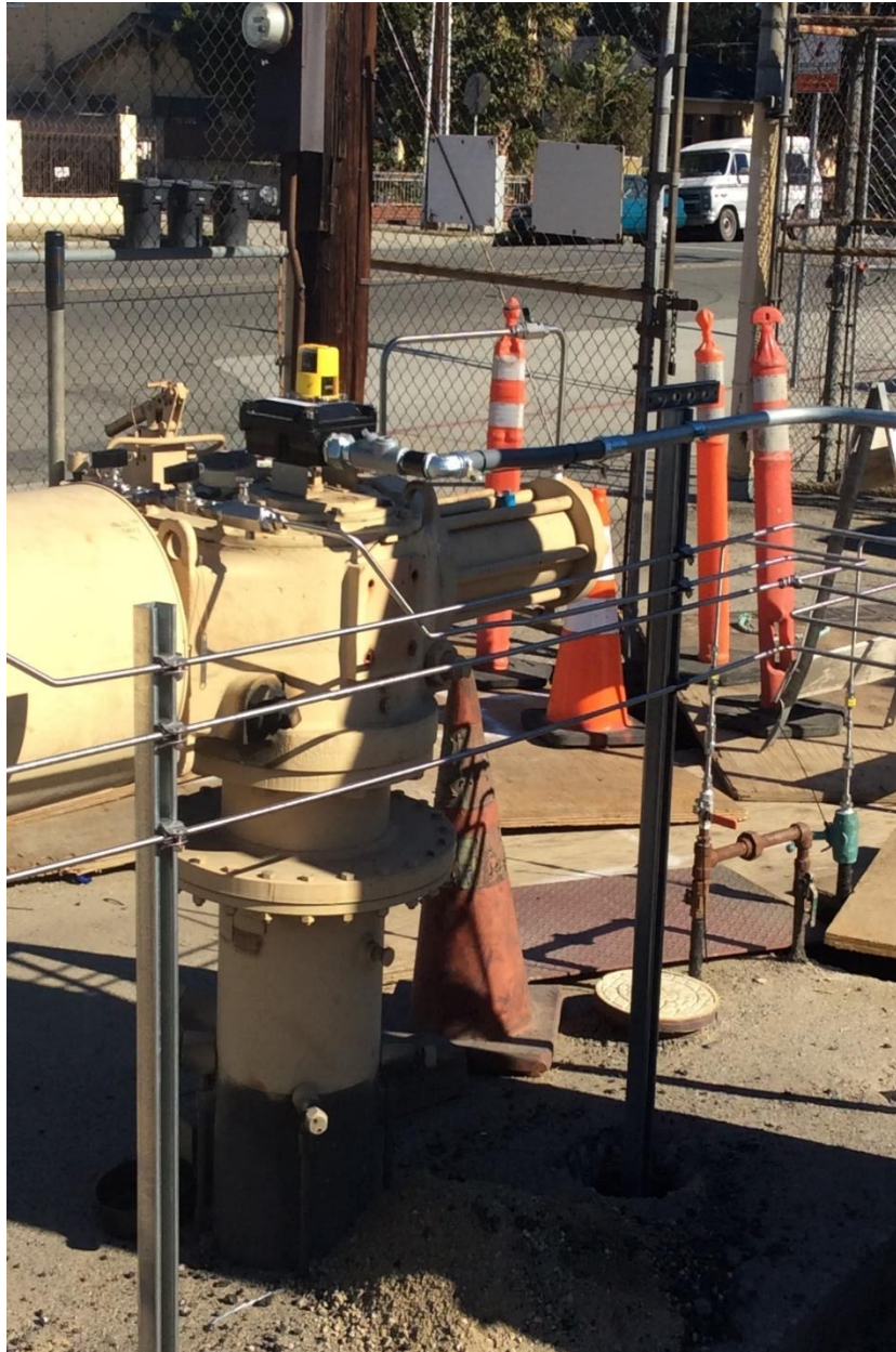
Figure 7: Salt Lake Station – Existing Actuator and New Instrument Gas Tubing
