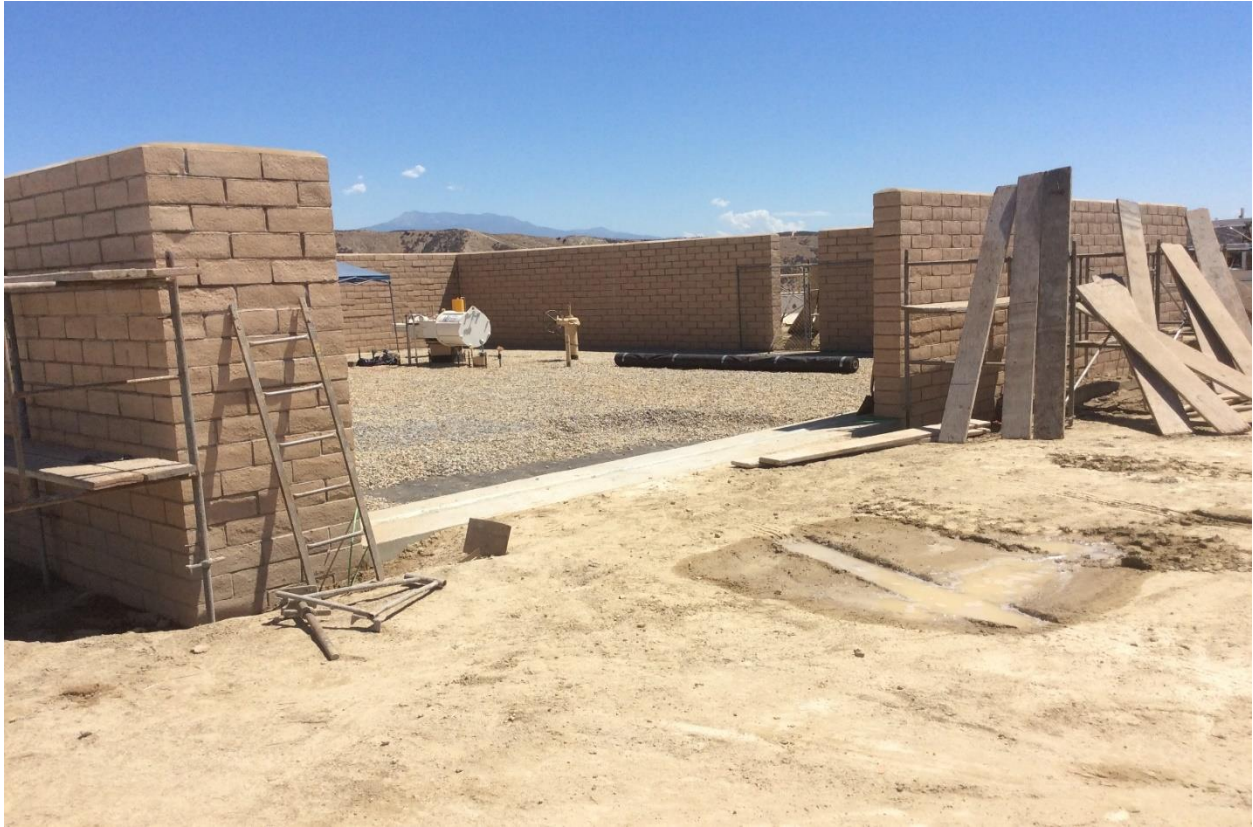
Figure 6: MLV 14.6B – New block Wall with the New Actuator in the Background
