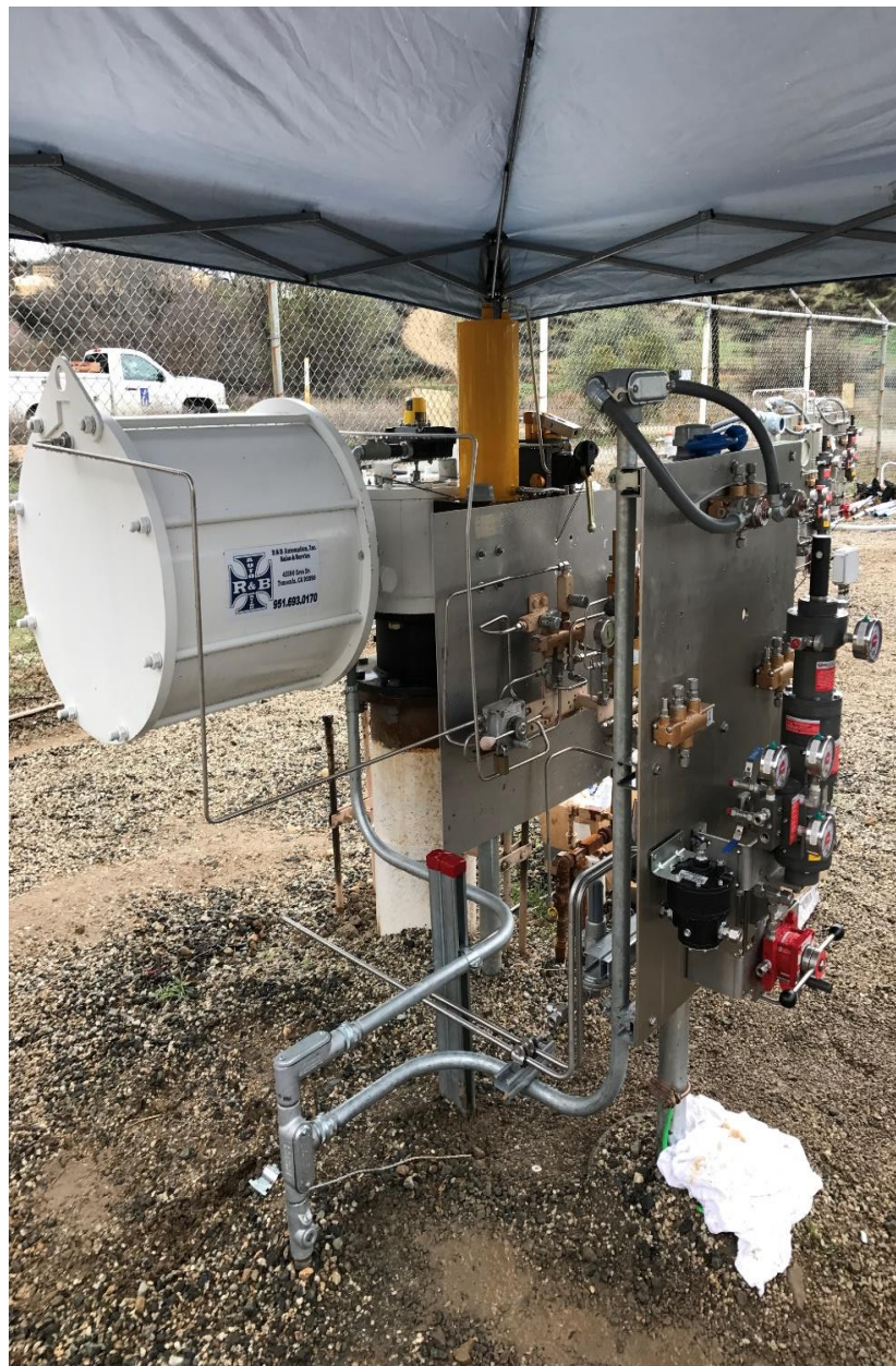
Figure 5: New actuator and Valve Regulating Pilots at Honor Ranch site
