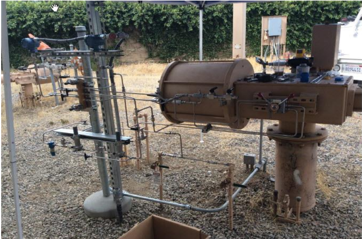
Figure 7: New Tubing and Three-Way Control Valve on Existing Actuator at Saugus Site
