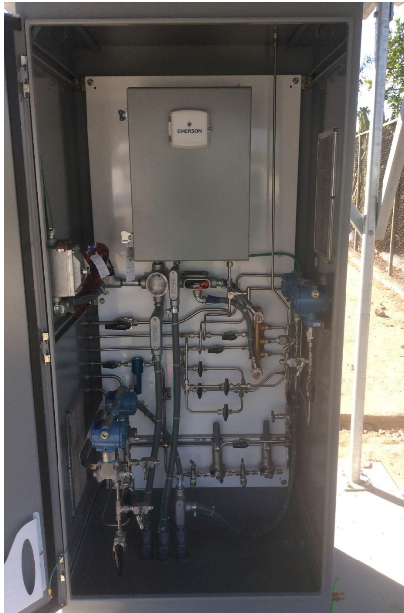
Figure 7: MLV 20 – New Linebreak Cabinet
