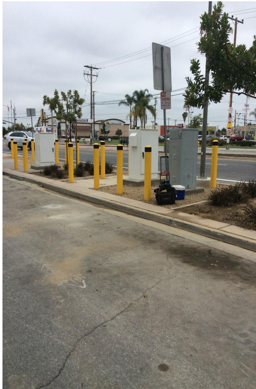
Figure 6: Central Avenue and 142 nd Street Project Site - Post Construction SCADA Cabinet and Battery Enclosure in Foreground, Linebreak Cabinet in Background
