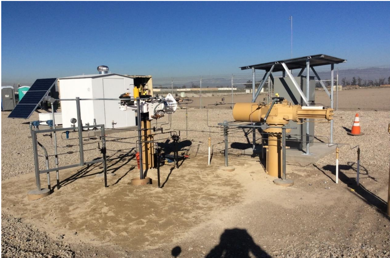
Figure 6: MLV 20A – Existing Actuator, New Actuator, Instrument Piping and New Linebreak Cabinet in the Foreground, New Electrical Shelter and Solar Array in the Background
