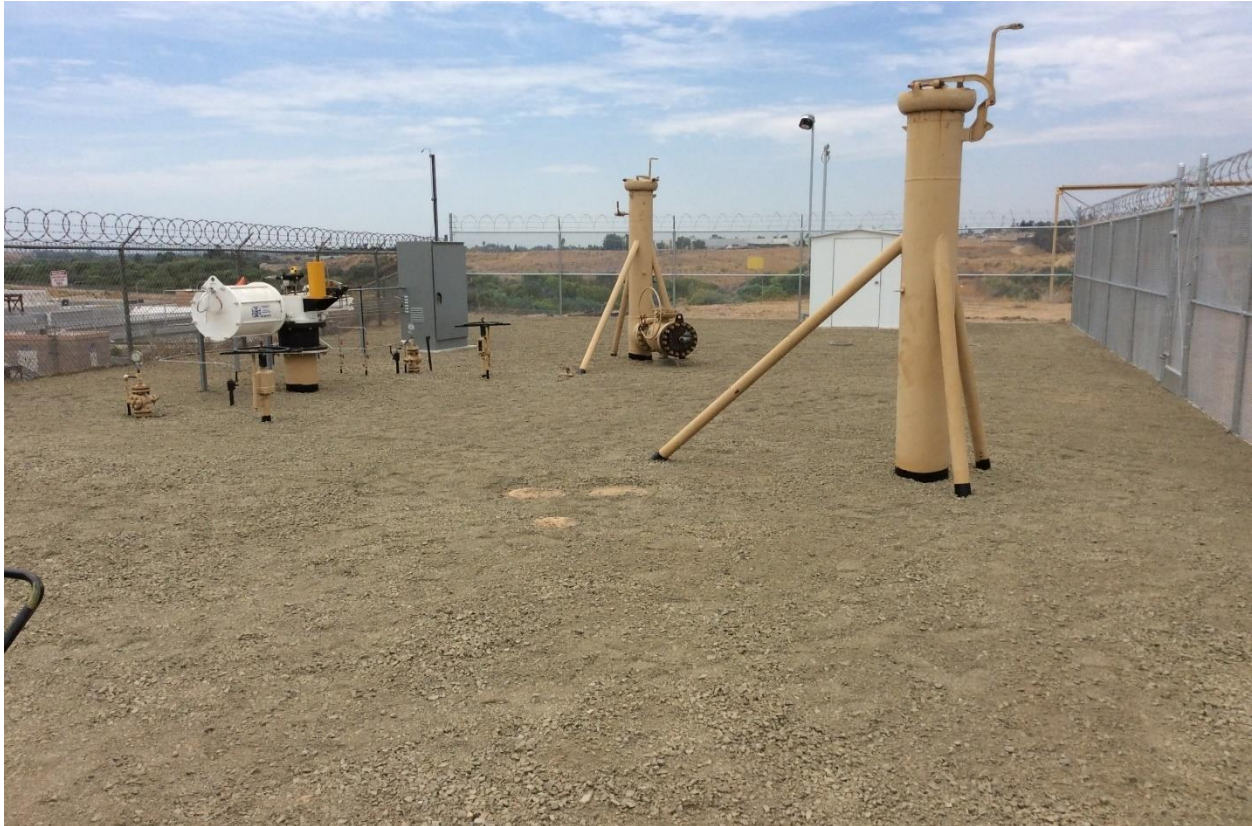
Figure 5: MLV 18A – New Actuator and Existing Blowdown Stack in the Foreground. Existing Blowdown Stack, New Linebreak Cabinet and New Electrical Shelter in the Background
