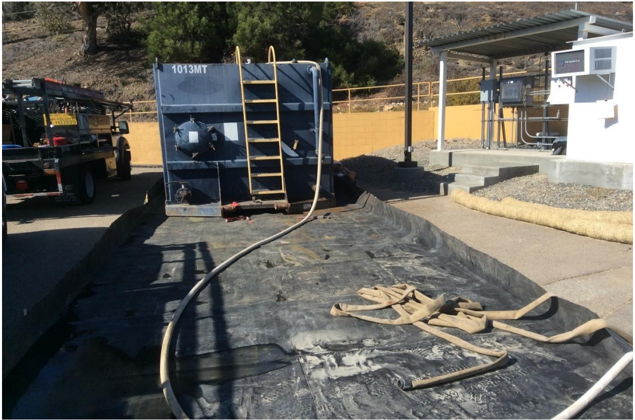
Figure 4: Temporary Storage Tank for Groundwater
