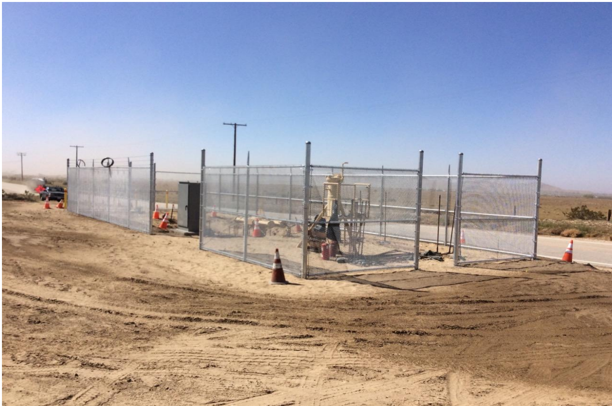
Figure 11: MLV 19A – New Fencing and Existing Blowdown
