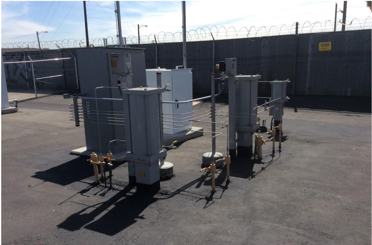
Figure 6: Slauson and Industry – New Actuators in Foreground, New Linebreak Cabinet and RCV Cabinet in Background
