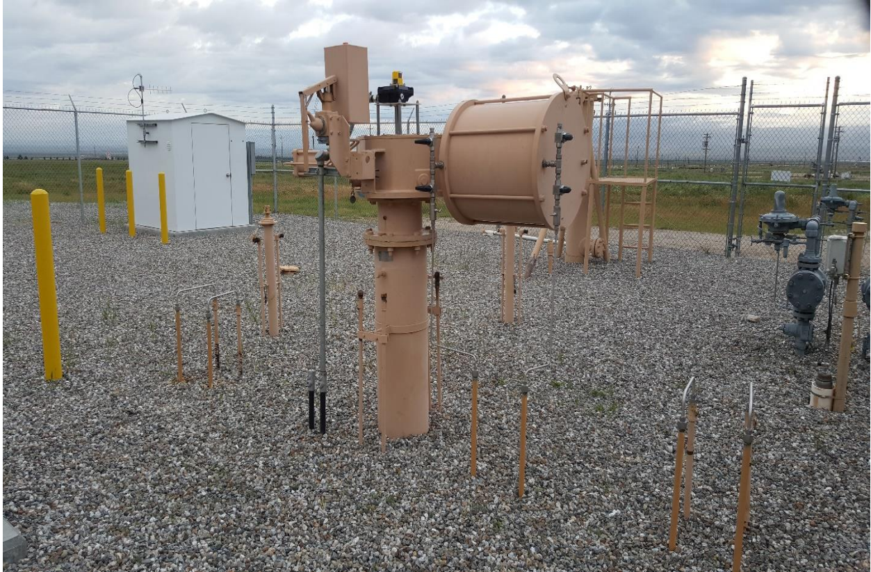
Figure 7: Laval Road – Actuator in Foreground, Shelter with Radio Antenna in Background
