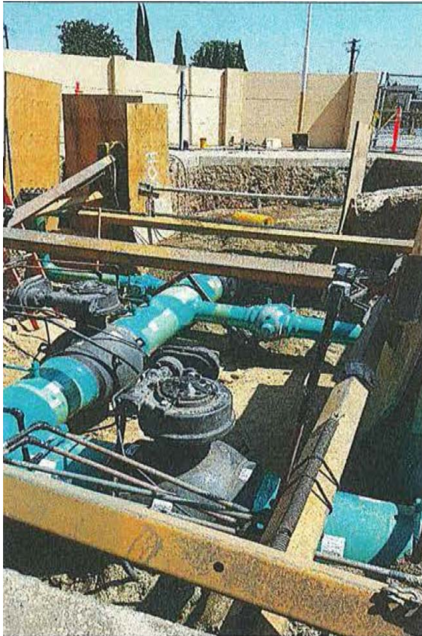
Figure 4: Alhambra Station Valve Enhancement Project – New Valve Assembly
