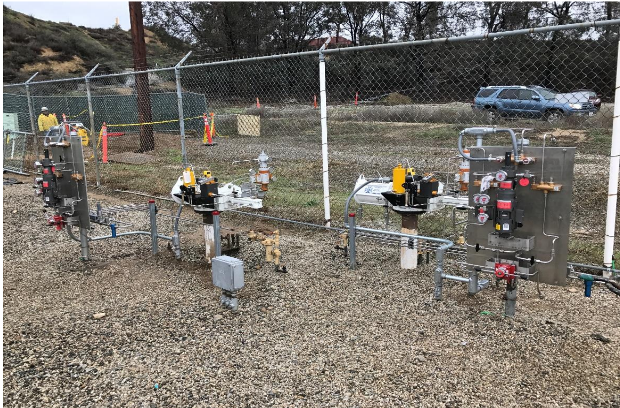
Figure 6: New Actuators and Valve Regulating Pilots on Bridle Valves at Honor Ranch Site
