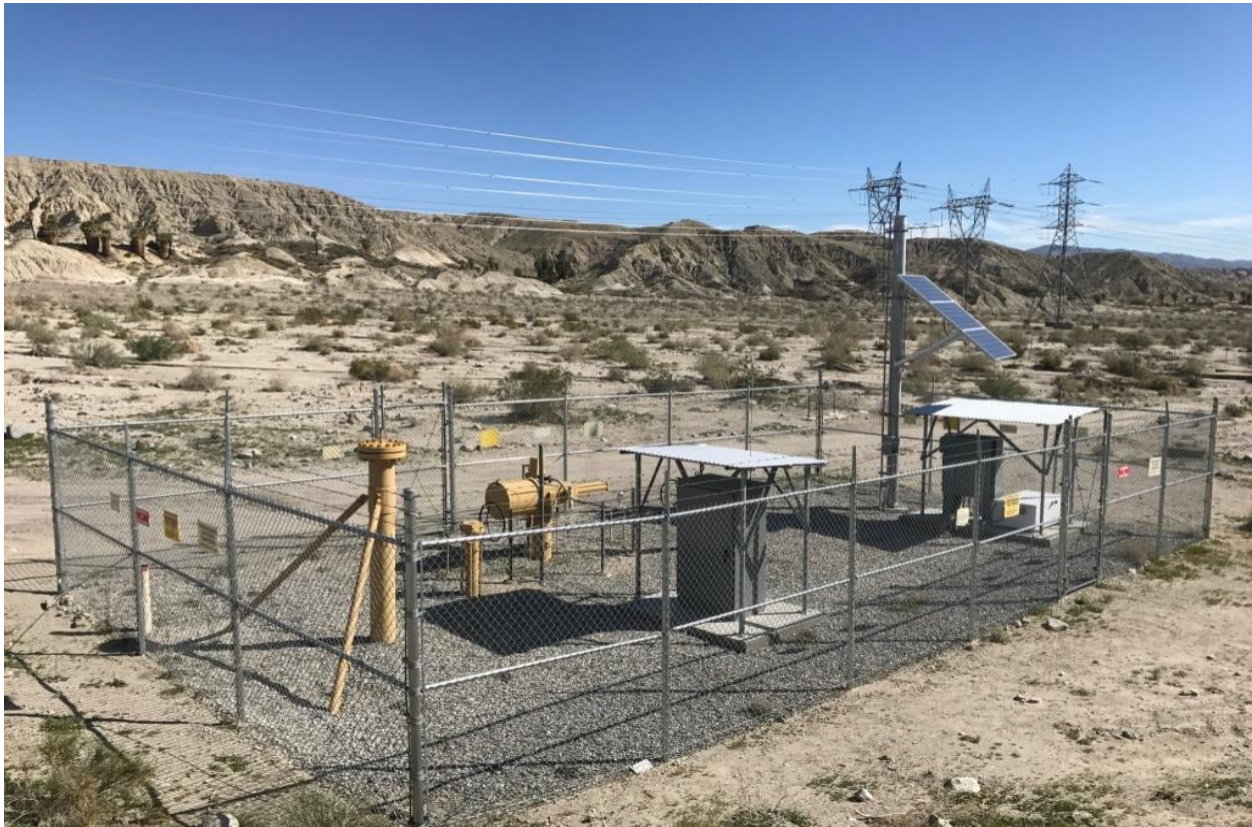
Figure 6: Valve 9 – Post Construction, Linebreak Cabinet in the Foreground, Shelter and Solar Array in the Background
