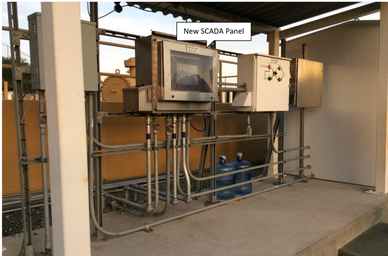
Figure 3: New SCADA Panel
