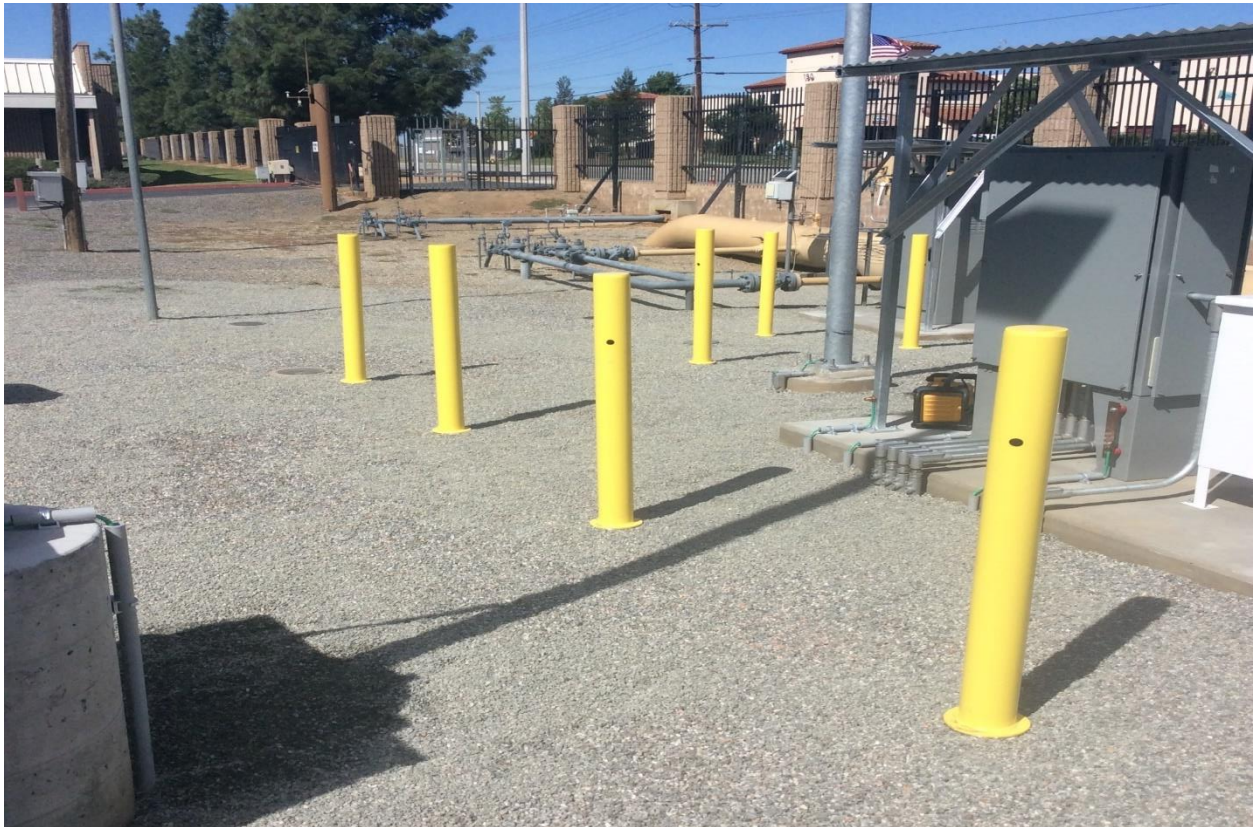
Figure 6: MLV 14 – New Supervisory Control and Data Acquisition (SCADA) Cabinet and Bollards
