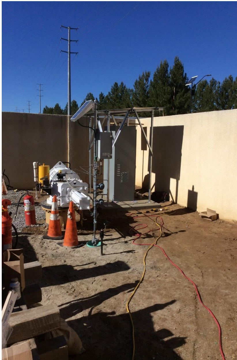
Figure 5: MLV 14B – Solar Panel and Actuator in Foreground, New Linebreak Cabinet and Canopy in the Background
