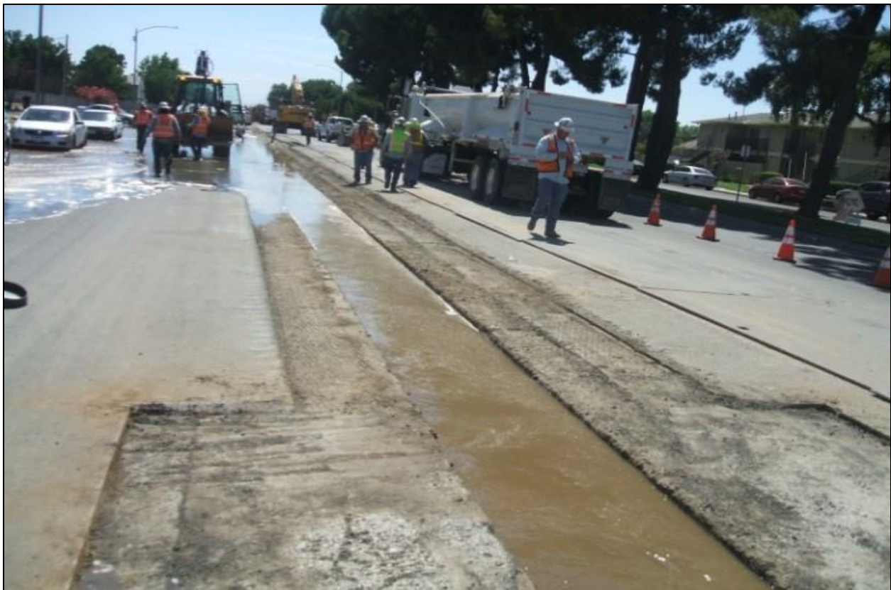
Figure 5: Section 2 - Broken Waterline
