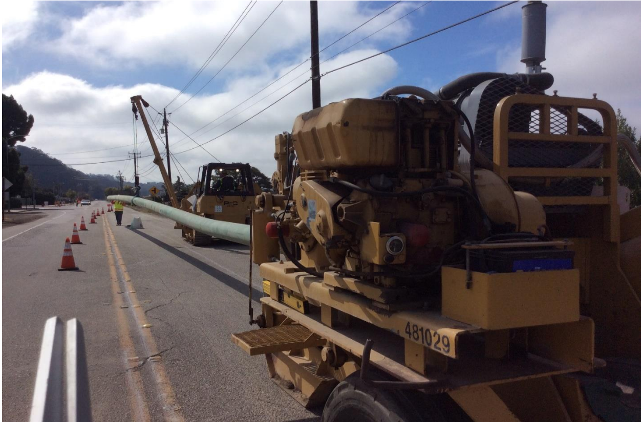
Figure 12: Section 7A – Removal of Pipe from a Bending Machine After Fabrication of a Sag Bend
