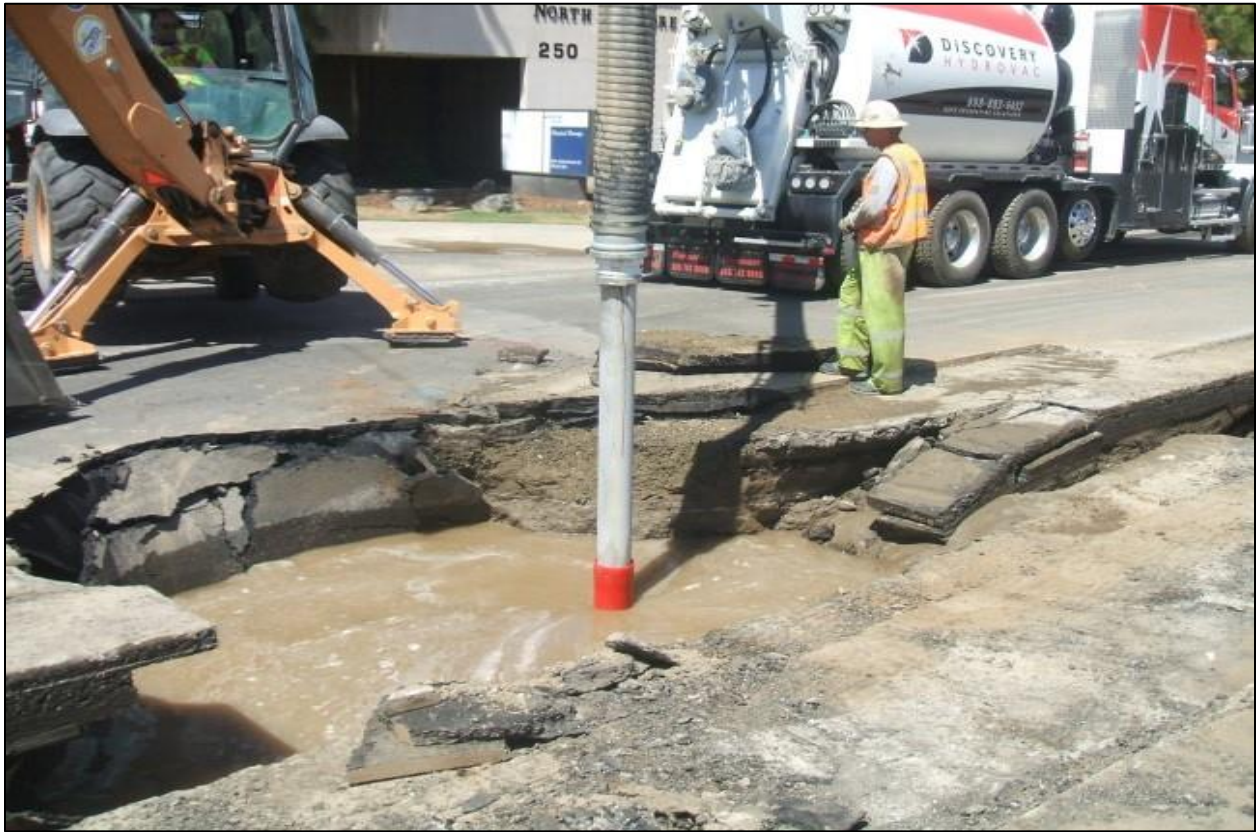
Figure 6: Section 2 - Broken Waterline Clean Up
