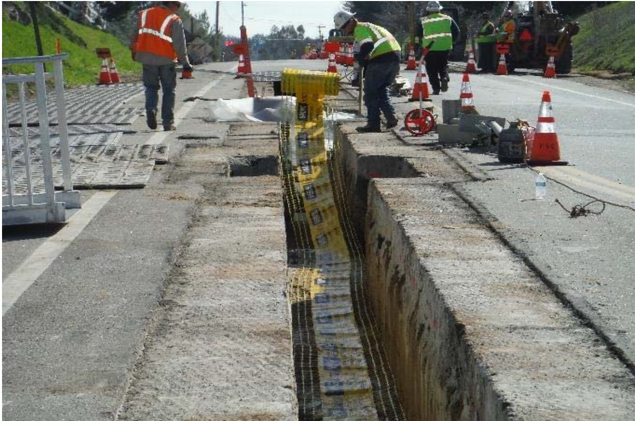
Figure 7: Safety Tape Over Pipe
