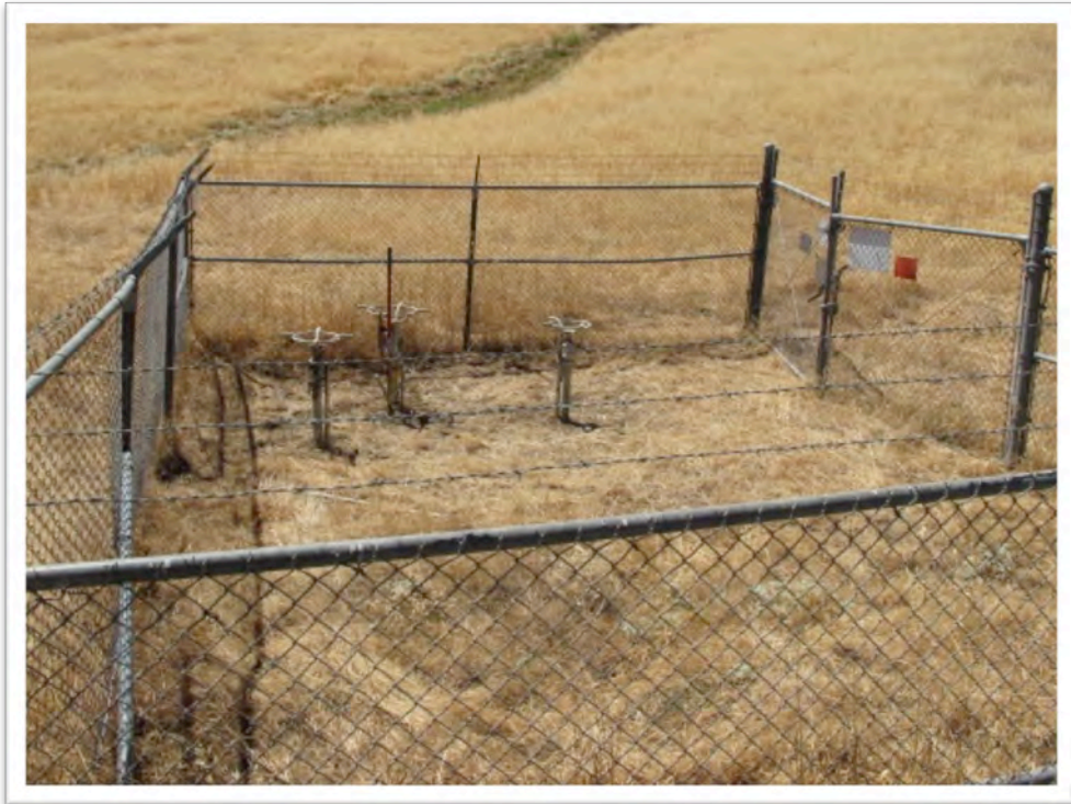
Figure 12. Mainline valve station for Line 306 at [REDACTED]
