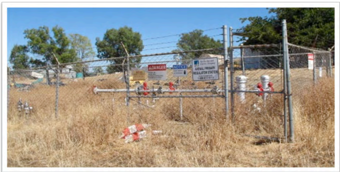
Figure 6. PG&E tap to City of Avenal near intersection of Hydril and Avenue 36.
