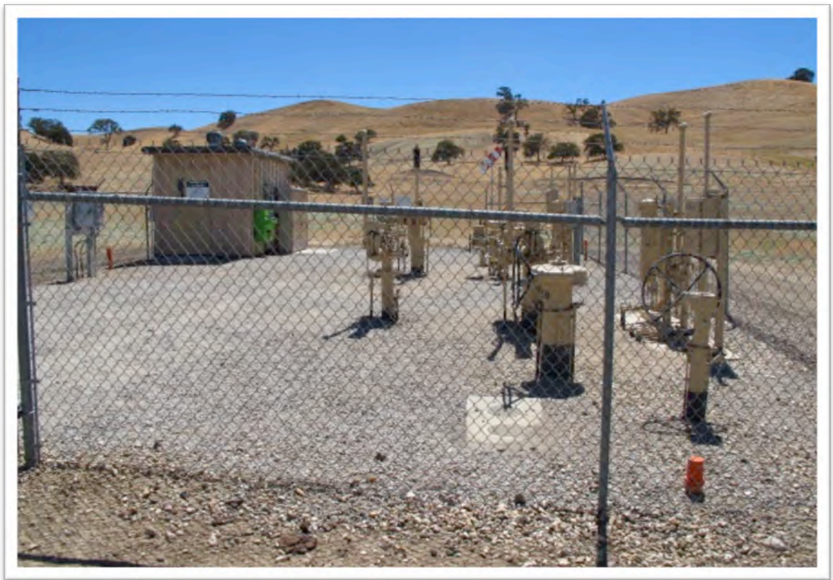
Figure 23. Another view of installation at Estrella Station at Mile Marker 40.30.
