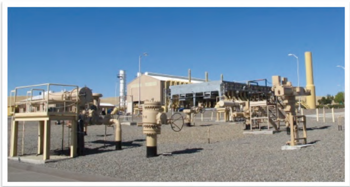
Figure 2. Compressor station facilities at Kettleman City Station (Avenal).
