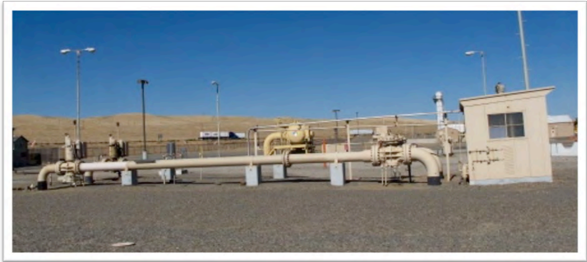
Figure 3. Feed off PGE A & B main line that feeds Line 306 from compressor back to this installation.
