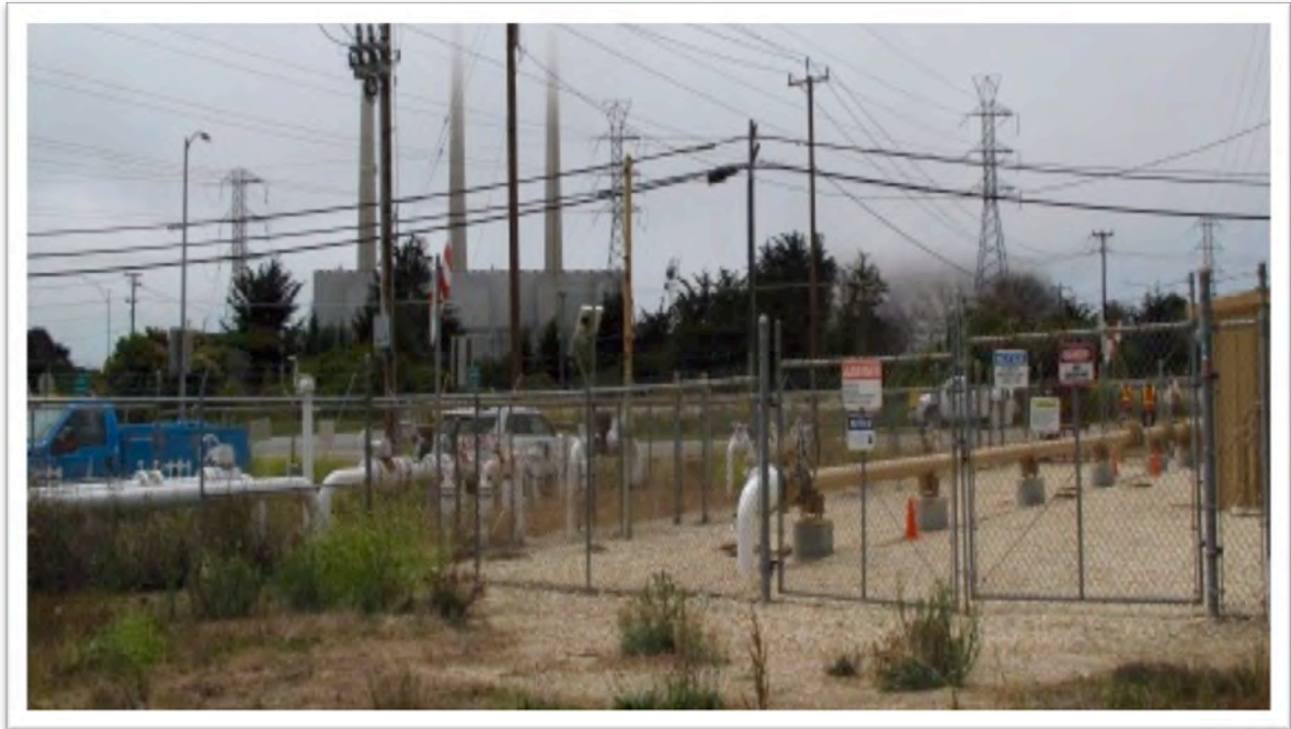
Figure 41. View of Morro Bay terminal and SoCalGas interconnect with inactive generation plant in background.
