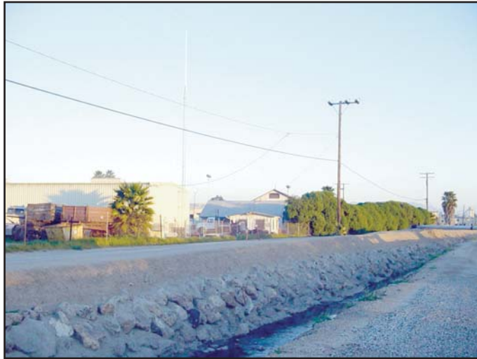
Photo 1 View of concreted rip-rap that lines the banks of Brown Barranca in the Satcoy District.
