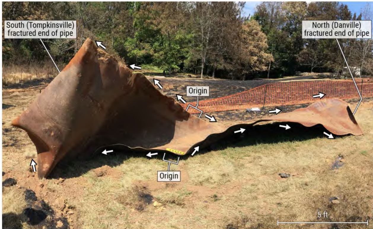
Figure 5. Ejected pipeline segment.
